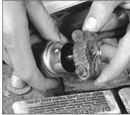
10.7a When cleaning the cable clamps, all corrosion must be removed (the inside of the clamp is tapered to match the taper on the post, so don't remove too much material)
