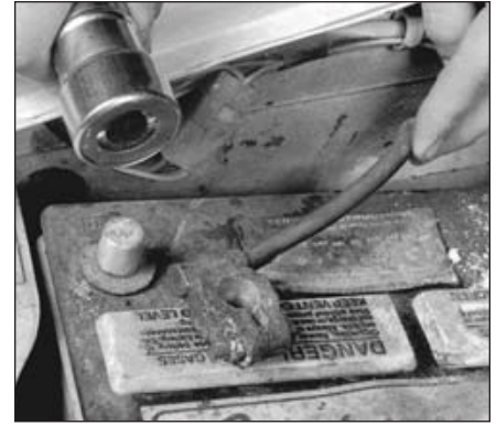
10.7b Regardless of the type of tool used on the battery posts, a clean, shiny surface should be the result
